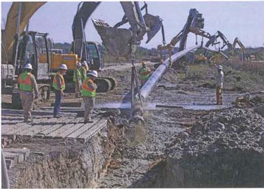
Figure 1. Delta Directional owner, Billy Cleveland (closest to pipe) watches as 6228 ft (1898 m) of natural gas pipeline is installed on Honey Island.
